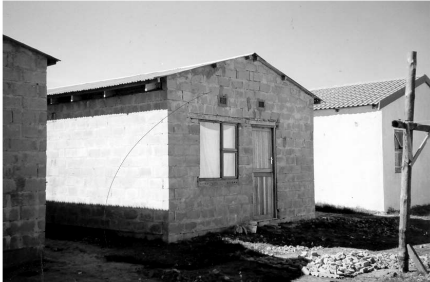
Fig. 1: Noma's house with some of the problems visible, area above the wall and below the roof not filled in, no ridge piece, bad workmanship above door and window.
